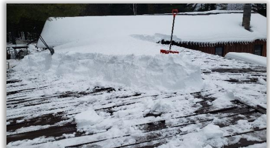
Up to 4 feet of snow on the Maintenance Shop roof!
